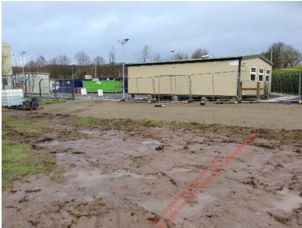
Figure 15.5 Temporary contractor's compound within garden shown on 1 st ed. OS map, looking NE.
