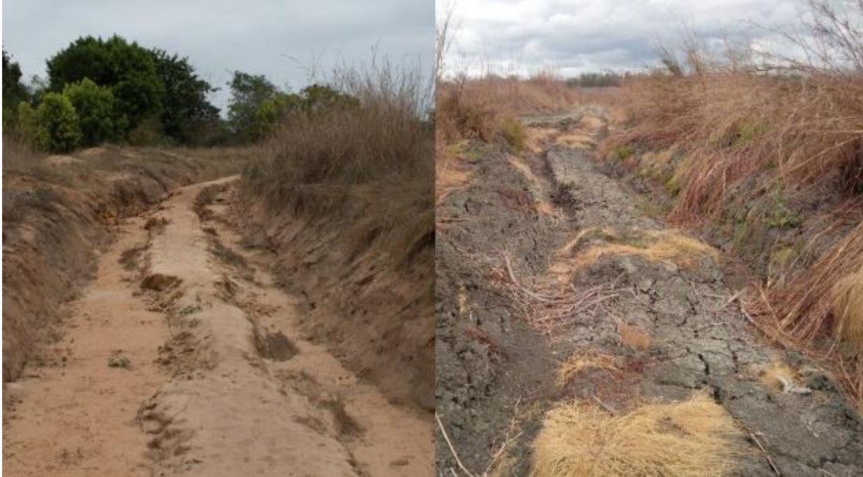
FIGURE 5 - SANDY (LEFT) AND "CATETE" CLAY (RIGHT) SOIL ROADS DEEPLY CARVED BY TRUCK CIRCULATION IN SOUTH EAST QUIÇAMA
