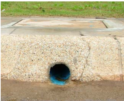
Stormwater draining to ocean
