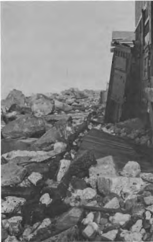
Figure 10. Wave damage to house at Redondo Beach. Photographed January 17, 1953, after a small storm.
