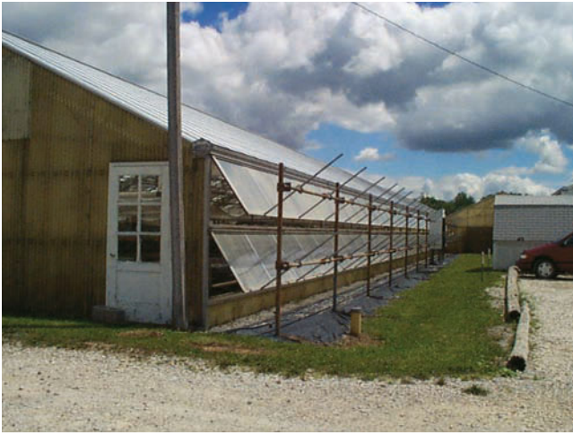
FIGURE 19-11. Side vents permit cool air to enter the greenhouse, forcing the hot air out through the top vents. (Delmar/Cengage Learning. Photo by Steven Newman.)
