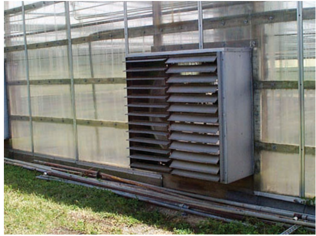
FIGURE 19-12. A greenhouse exhaust fan (Delmar/Cengage Learning. Photo by Steven Newman.)
