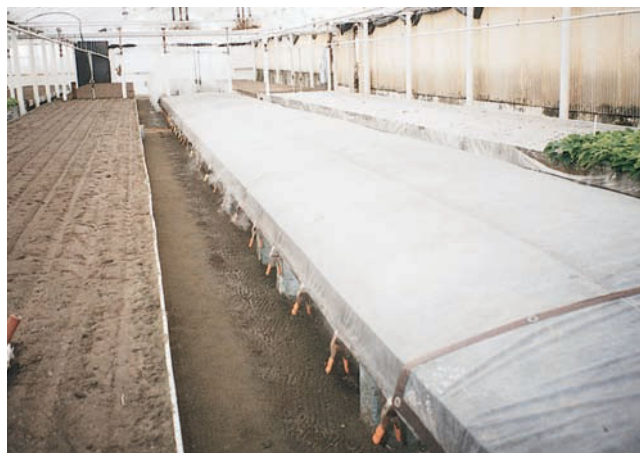
FIGURE 20–1. This greenhouse ground bed is being steam pasteurized. A tarpaulin held down by clips prevents the steam from escaping. (Delmar/Cengage Learning. Photo by Steven Newman.)
