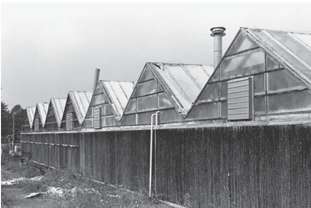
FIGURE 19–16A. In this pad and fan cooling system, continuously wet pads of excelsior cool the air drawn through them into the greenhouse. (Delmar/Cengage Learning. Photo by Jack Ingels.)
