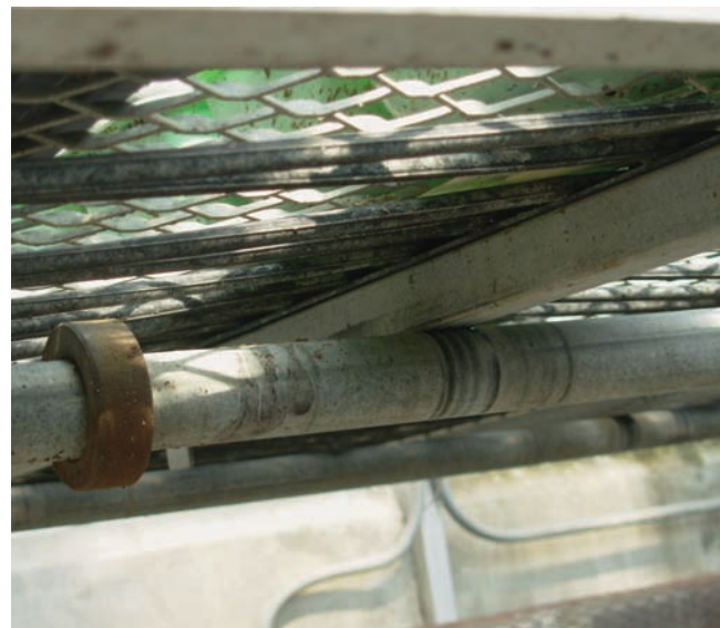
FIGURE 19-24B. The rolling pipe system beneath a bench (Courtesy of Robert Sutherland)
