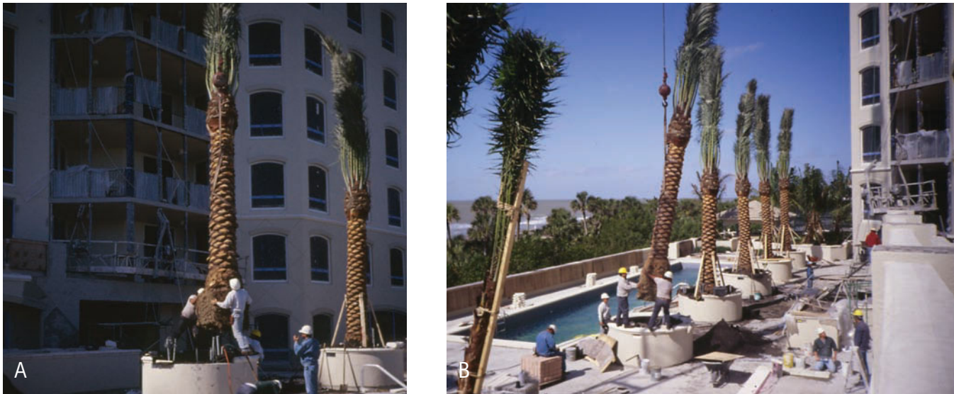
FIGURE 10-16A and B. Large palms, with fronds tied, are set into planters using a crane. (Delmar/Cengage Learning. Photo by Jack Ingels.)
