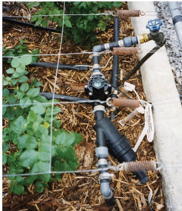
FIGURE 20–11. A semiautomatic irrigation system used in a ground bed for watering roses. Note the control valve, the pipes along the side of the bed, and the ooze tubes crossing the bed at intervals. (Delmar/Cengage Learning. Photo by Jack Ingels.)
