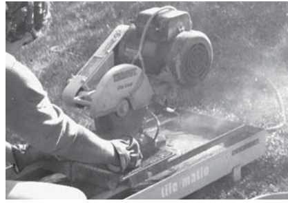
FIGURE 17-8. A landscaper using a tile saw to cut pavers for a patio. (Delmar/Cengage Learning)
