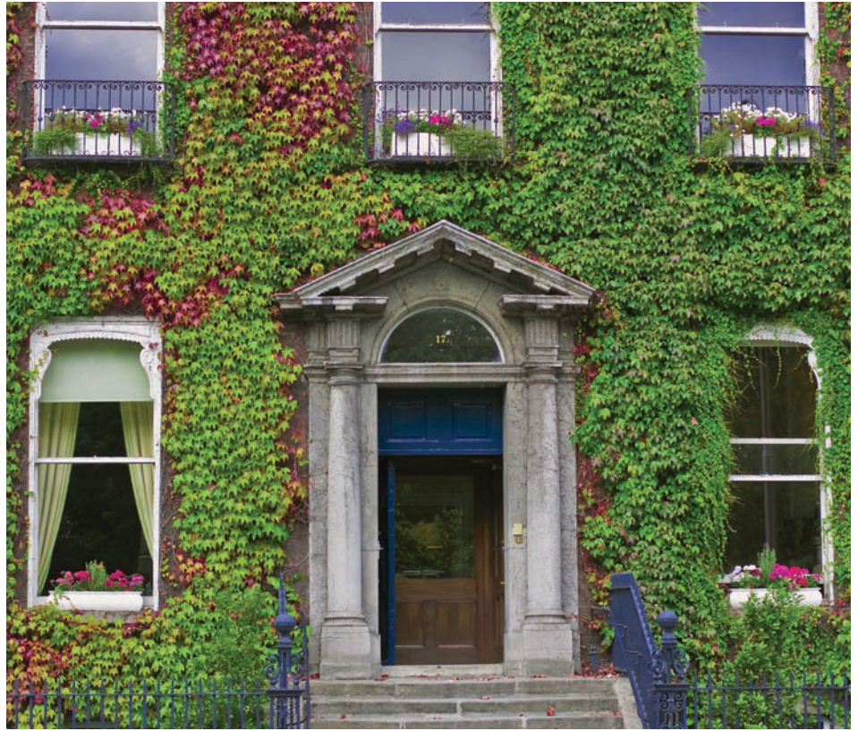
FIGURE 12–2. Vines contribute an architectural quality to this building. Regular maintenance is required to keep the windows and shutters from being overgrown. (© Nathan Guinn, 2009. Used under license from Shutterstock.com)
