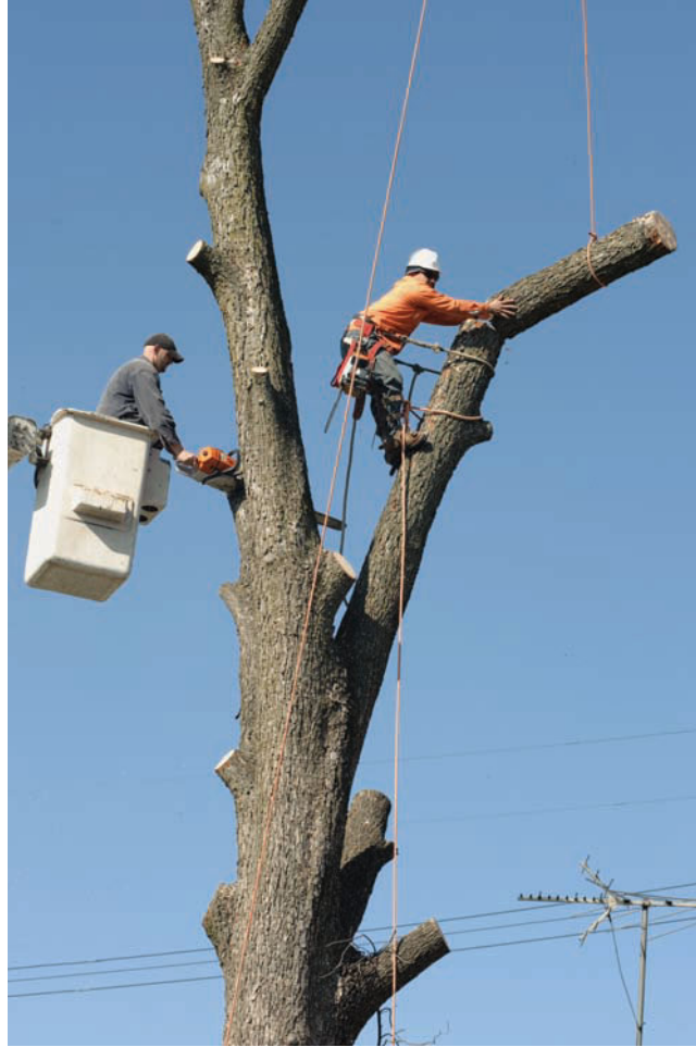
FIGURE 18–3. Careful use of ropes permits this arborist to remove a dead tree next to a busy street with minimal danger or disturbance to passing people or traffic. Tree removal is only one of the many tasks performed by professional arborists. (© Randy Mirmontez, 2009. Used under license from Shutterstock.com)
