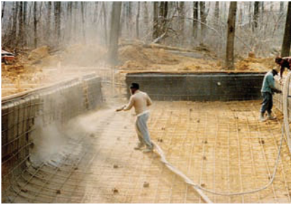
FIGURE 17-7. A landscape subcontractor applies sprayed concrete to the walls of a swimming pool. (Delmar/Cengage Learning)
