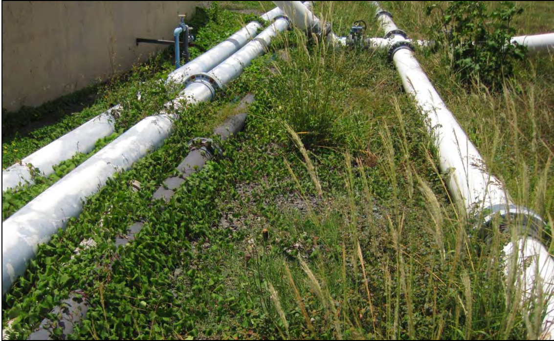
Figure 28. Photograph showing piping extending between Kāne‘ohe WWPTF tanks, view to west
