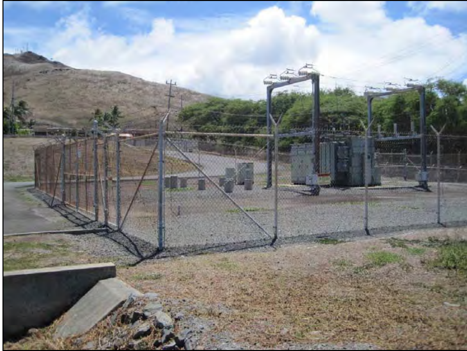
Figure 41. Overview showing location of “Facility 1” at the Kailua WWTP, view to west
