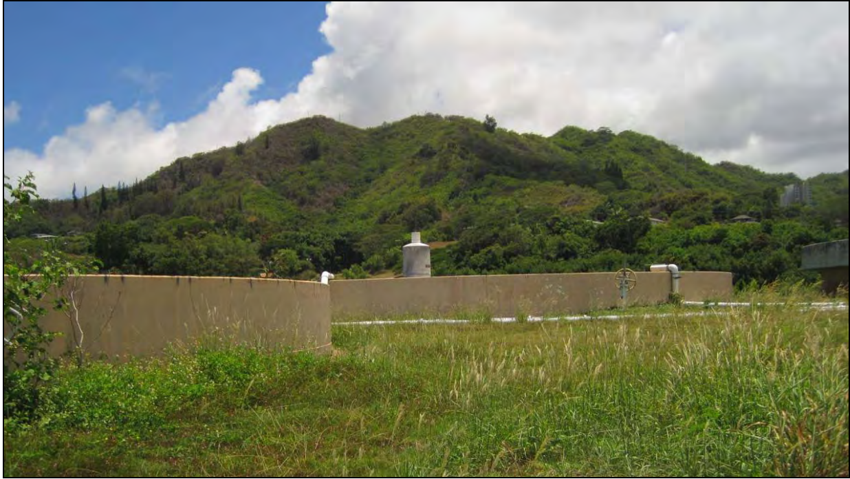
Figure 26. Photograph showing large holding tanks where improvements are planned in central portion of the Kāneʻohe WWPTF, view to southeast
