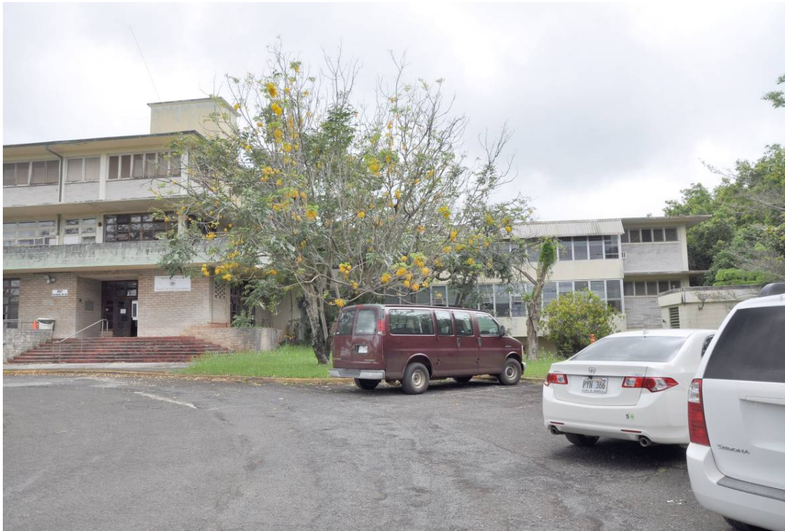
The two building wings east of the main lobby (right) have only two levels.
