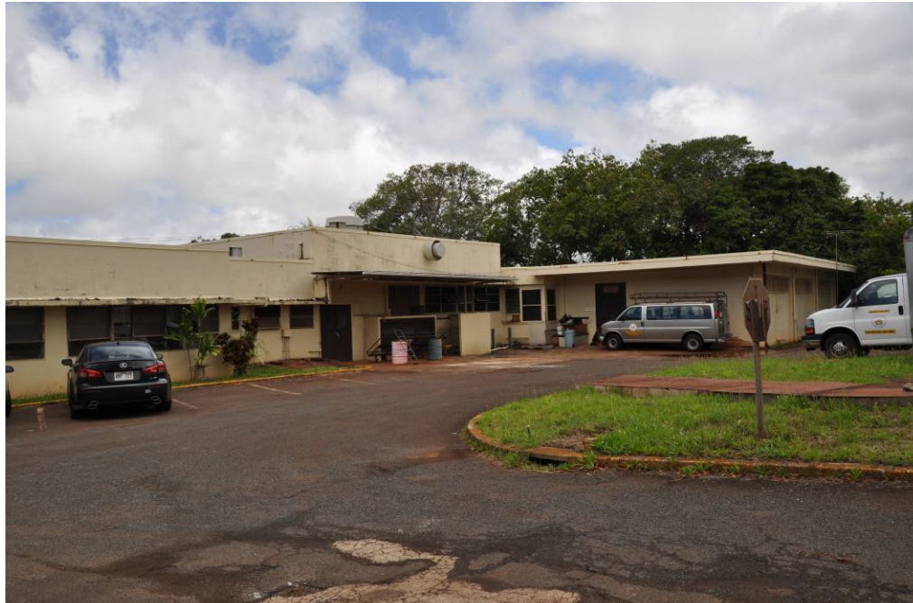
The Kitchen and Dining building is not eligible for listing on the National Register of Historic Places as a stand alone structure, but is eligible as a contributing structure to the Waimano Home hospital site.
