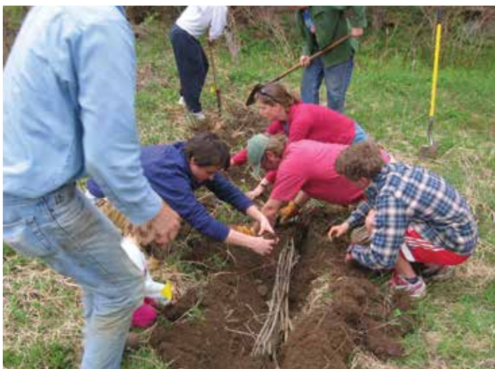
Community volunteers install willow wattles to stabilize the bank along the North Branch of the Winooski River.
