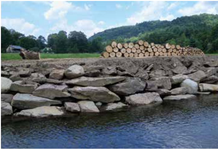
Trees along the bank of the Ompompanoosuc River were cut and replaced with rock riprap—a move in the wrong direction toward establishing equilibrium.
