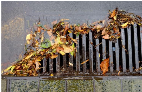
Figure 70 - Organic debris in storm drain
