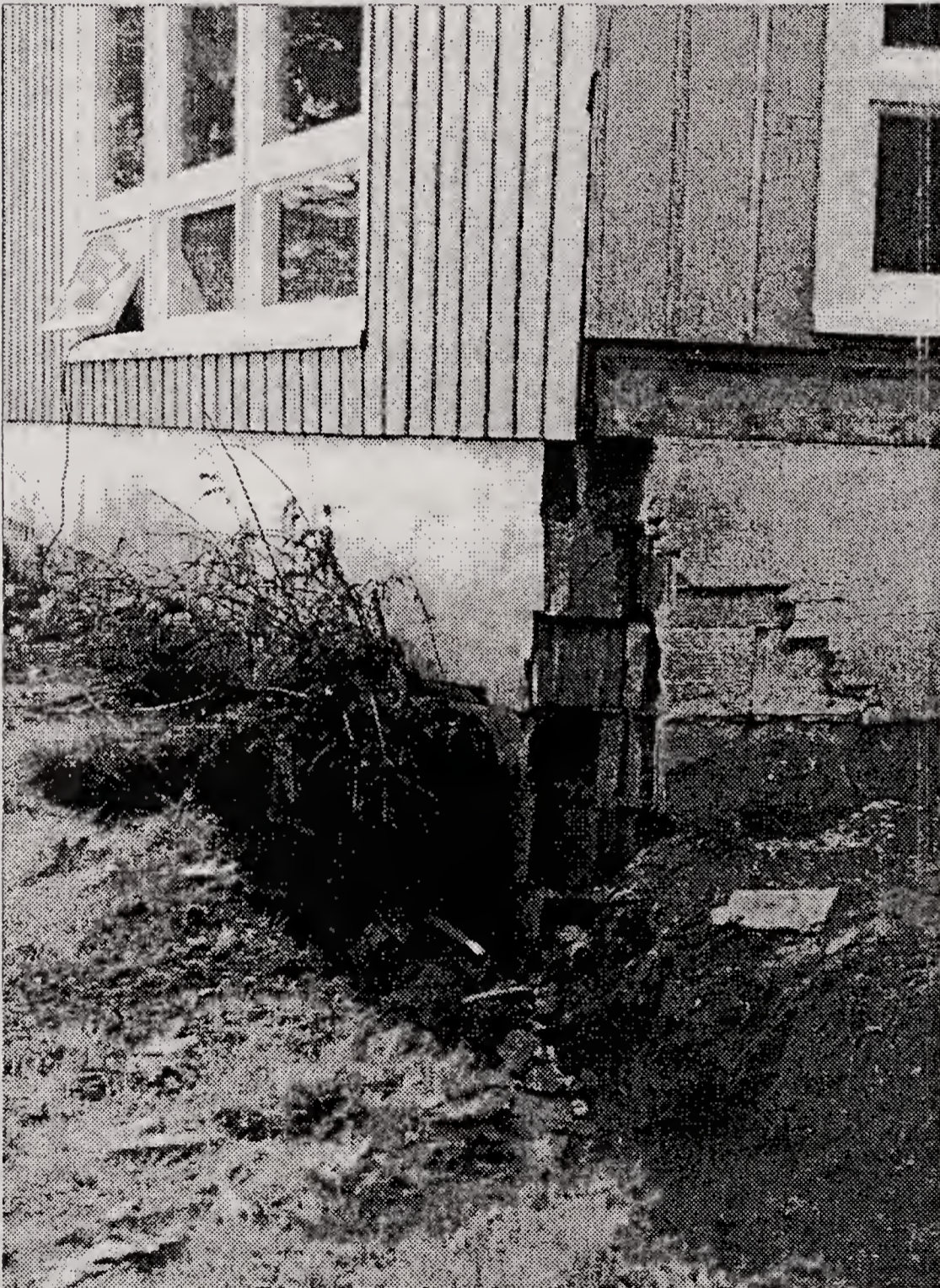
Work in progress. Note the badly damaged concrete blocks. Photograph by Howard Chittenden.
