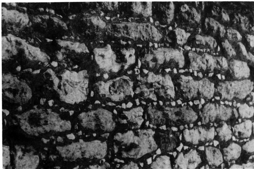
Fig. 6 Malmstone wall galleted with malmstone. Boundary wall at Old Hunstanton, Norfolk (TF 687 423)
