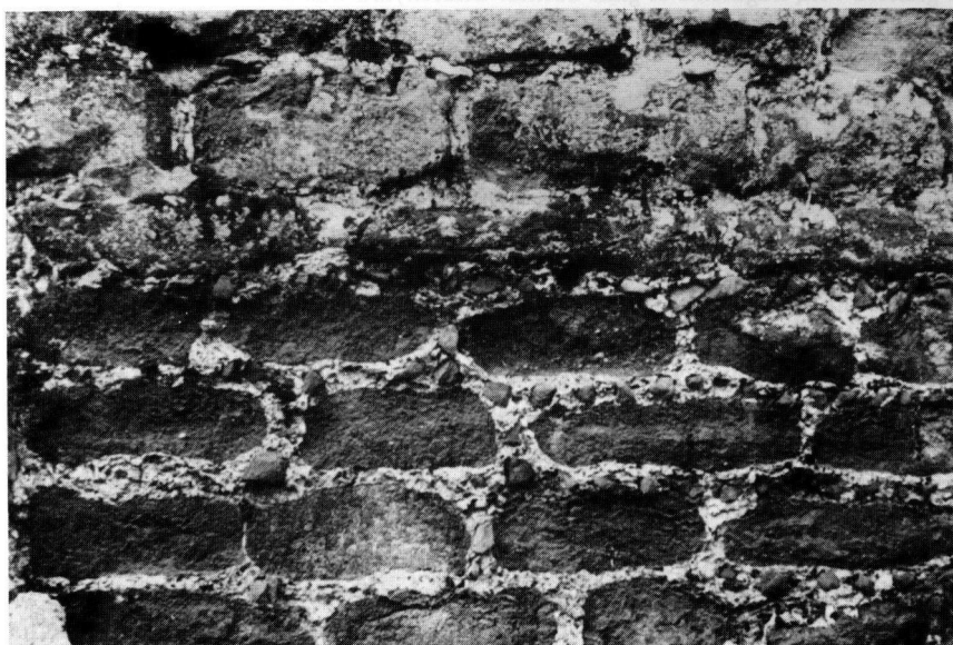
Fig. 11 Carstone wall galleted with fragments of brick. Boundary wall at Heacham, Norfolk (TF 675 373)
