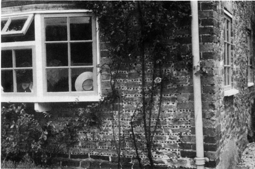
Fig. 2 Sandstone (Bargate) wall galleted with carstone. Cottage in Lower Eashing, Surrey (SU 945 437)
