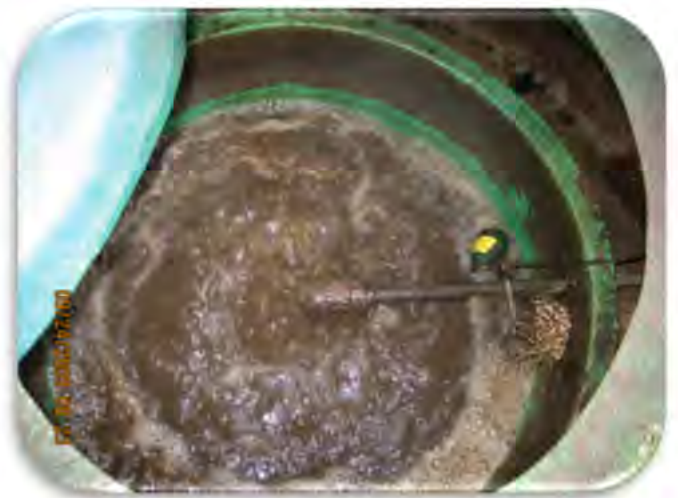
Figure 4. Aeration in an ATU.
