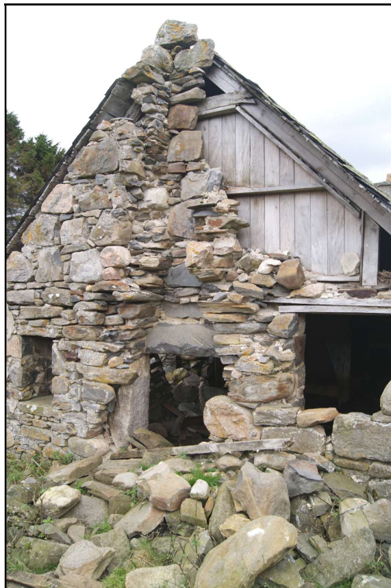
Shot looking at the collapsed SW gable
