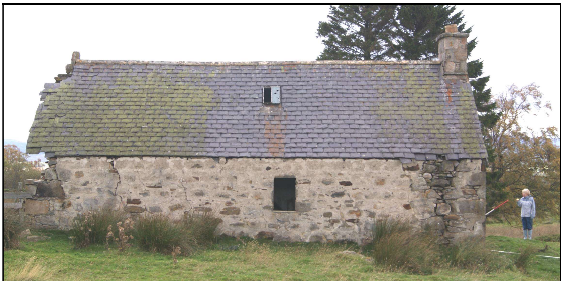
The SE wall showing the S corner which will soon collapse
