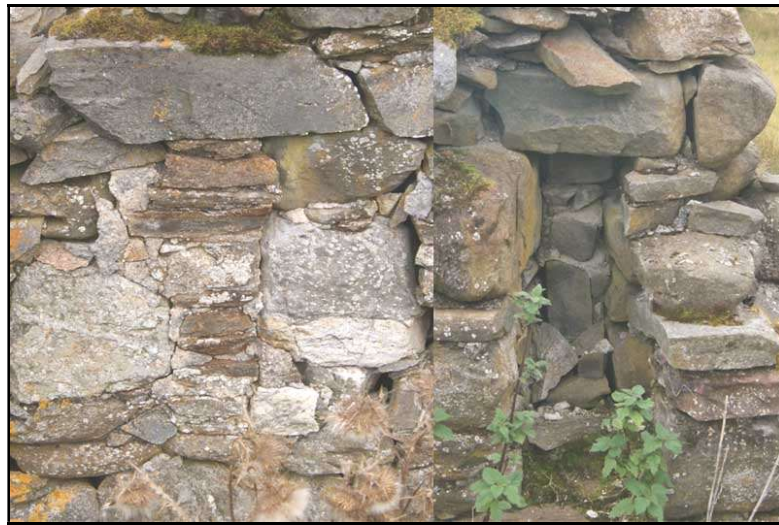
The two opposing slots for a possible central division, one blocked, the other not.
