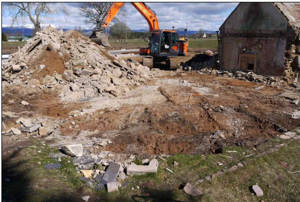
Figure 9 – Final ground level clearance of the croft building in progress. Facing N. Scales 1m
