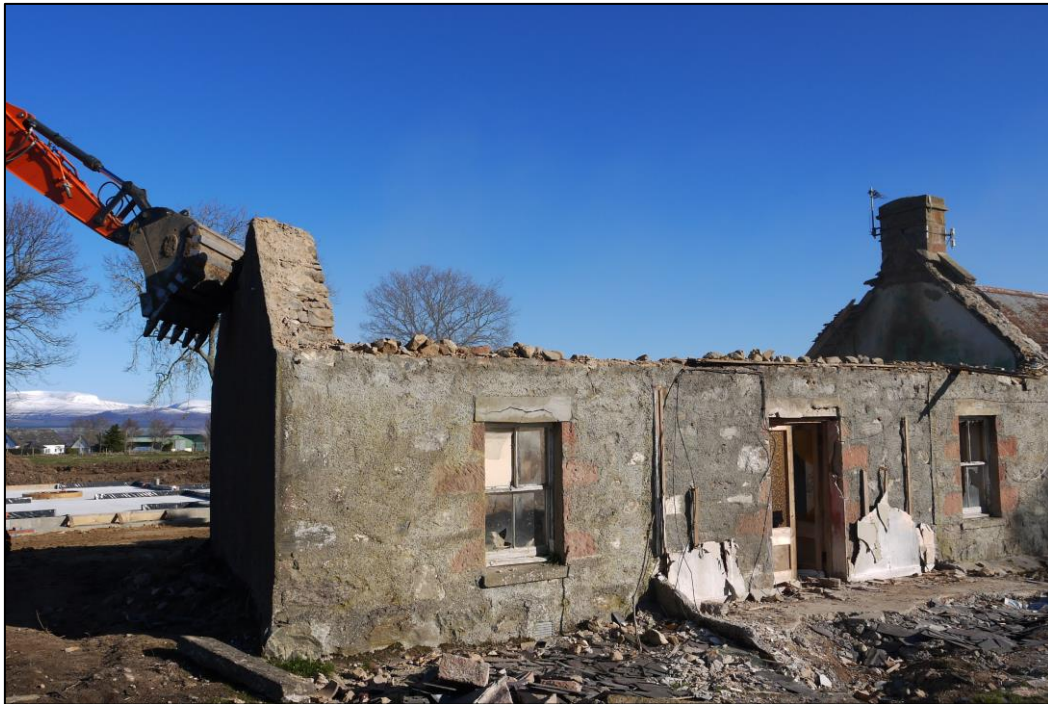
Figure 8 – Demolition of the croft building after removal of the roof structure. Facing N
