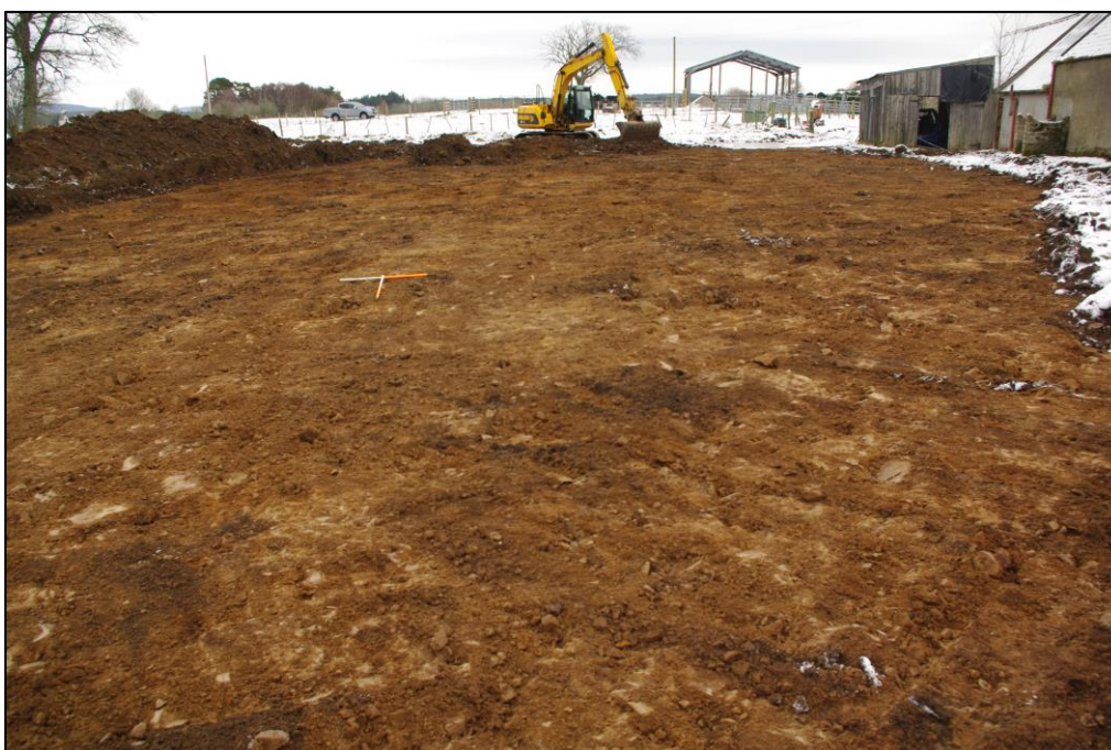
Figure 6 - The area of the new building after topsoil stripping. Facing NE. Scales 1m
