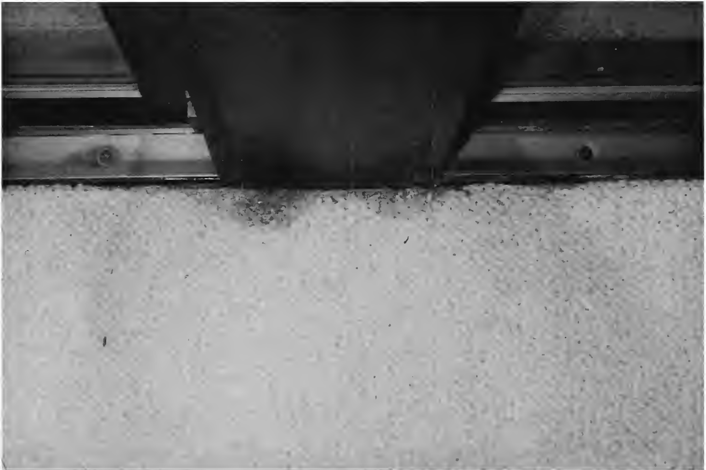
Figure 3. Photograph shows damage caused by plaster bagworm to edge of carpet adjacent to a sliding glass door.
