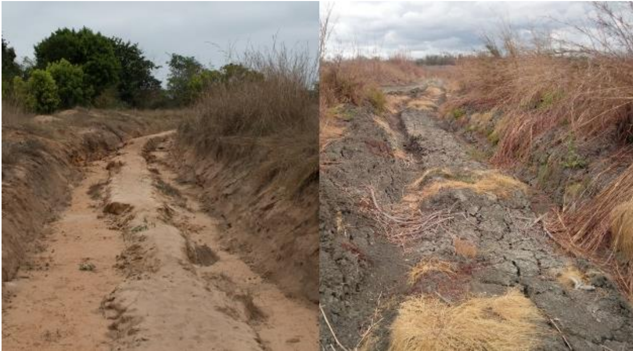
FIGURE 5 - SANDY (LEFT) AND "CATETE" CLAY (RIGHT) SOIL ROADS DEEPLY CARVED BY TRUCK CIRCULATION IN SOUTH EAST QUIÇAMA
