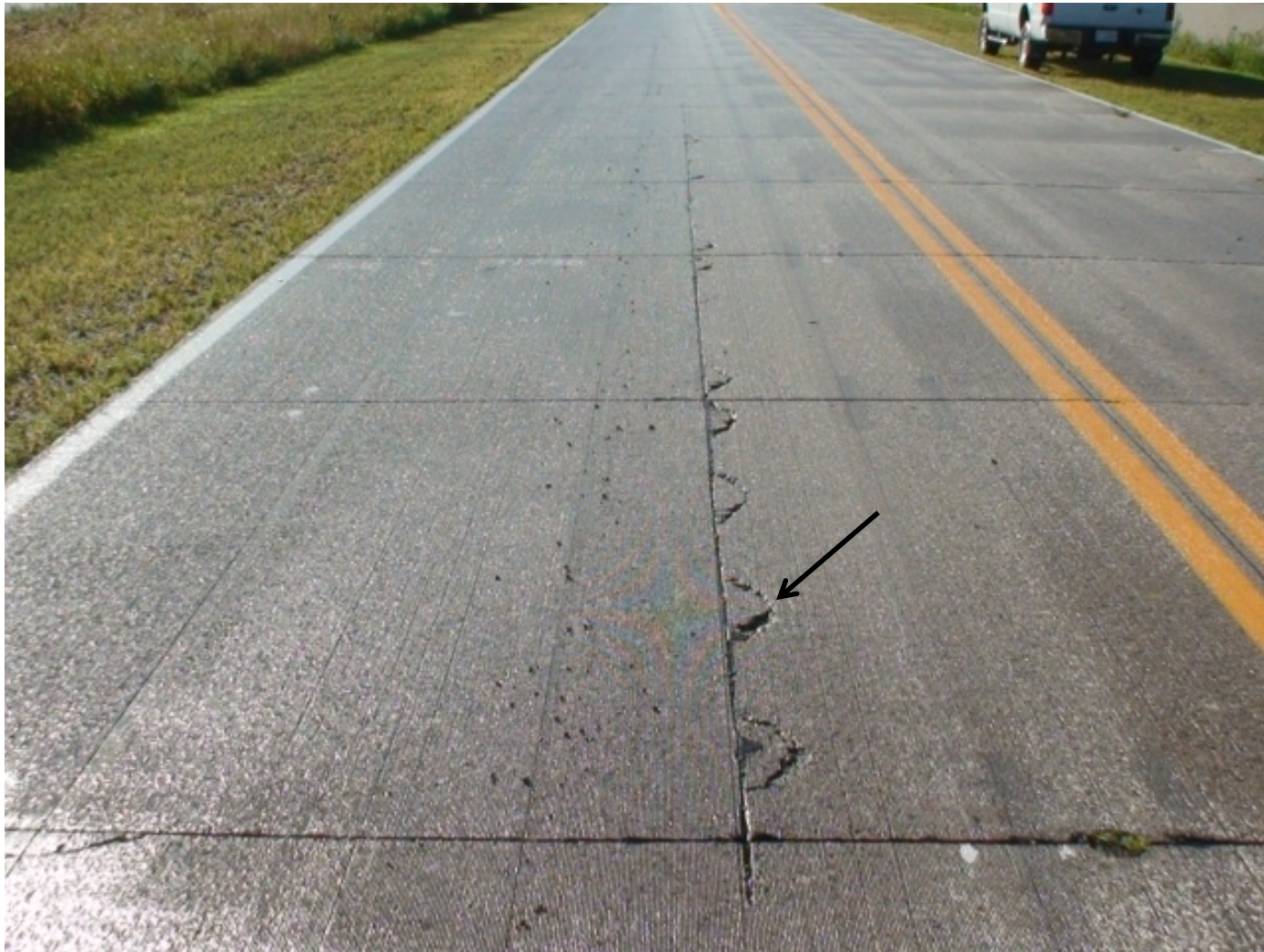
Plate dowels “popping through” longitudinal side of repair joints
