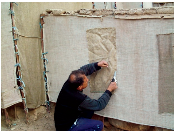
Figure 13. Patches on panels.
