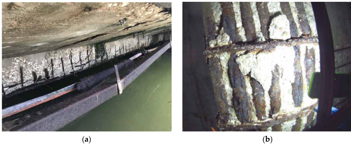
Figure 5. Picture of the bridge, showing significant corrosion: (a) lateral view of the deck and (b) view of the intrados of the beam.
