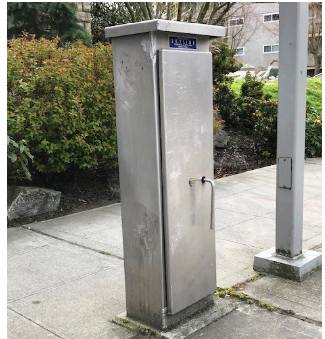
Power Pedestal at a Bus Stop
