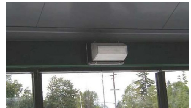
Standard Lighting Fixture in a Standard Shelter
