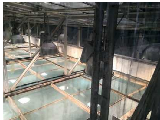
Fig. 11. Exterior of the diffusing ceiling with the lighting devices
