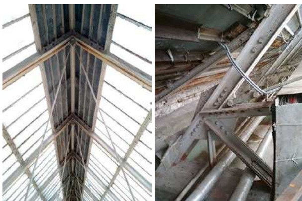
Fig. 8. Ridge of the lantern light transparent structure and traces of repairs
