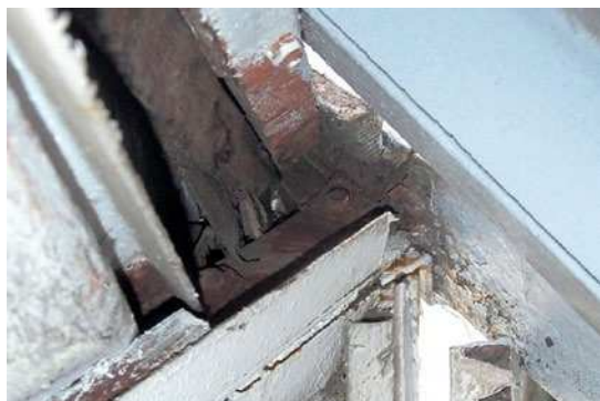
Fig. 4. Roof beam joint with traces of corrosion
