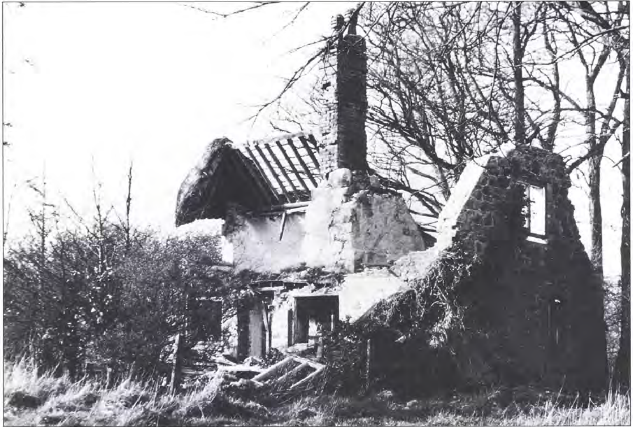
Plate LXV Old Totterdown Cottage collapsing in 1959 (now completely ruinous and overgrown)
