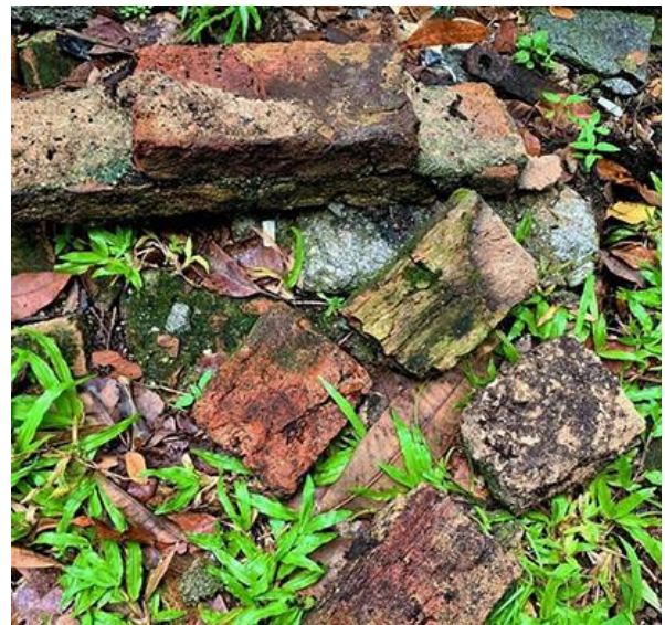
Fig. 2. Handmade bricks strewn on a grass patch below the cemetery wall, possibly dislodged due to weathering. Note their inconsistent shapes, sizes, textures and colours. (Photograph by: Lau Wing Lup).
