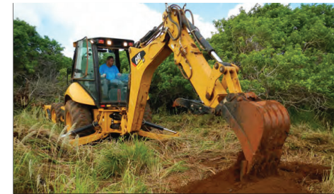
Figure 77: Excavation of Test Pit 21, looking southeast. The backhoe operator is Terrence Sarme.
