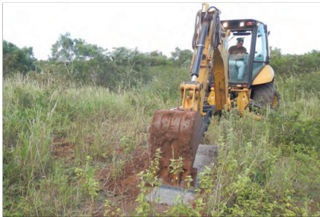
Figure 83: Excavation of Test Pit 24, looking south. Note the asphalt under the backhoe bucket. The backhoe operator is Terrence Sarme.
