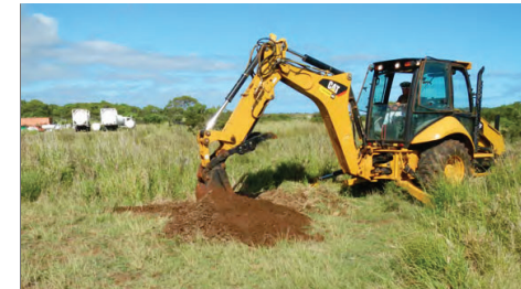
Figure 85: Excavation of Test Pit 25, looking southwest. Note the propane gas tanks in left background.
