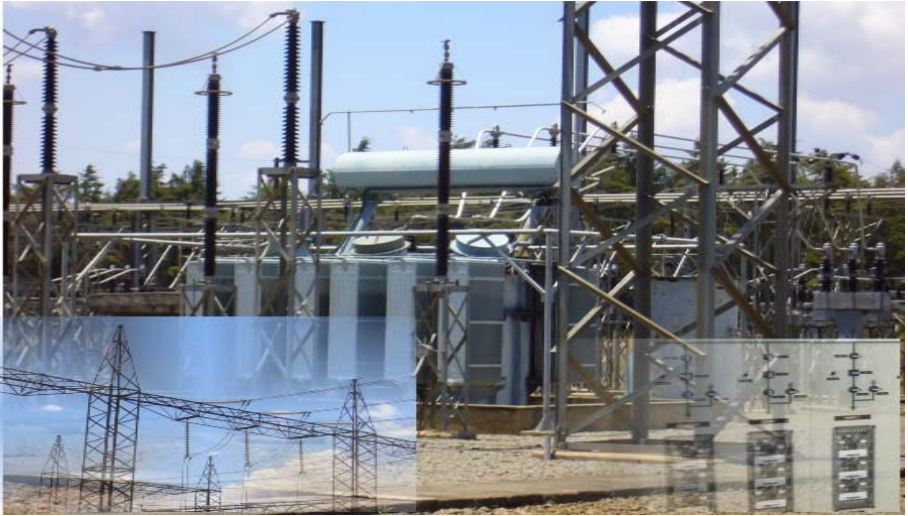
TANESCO Mwakibete Sub-station 220/33KV in Mbeya City
