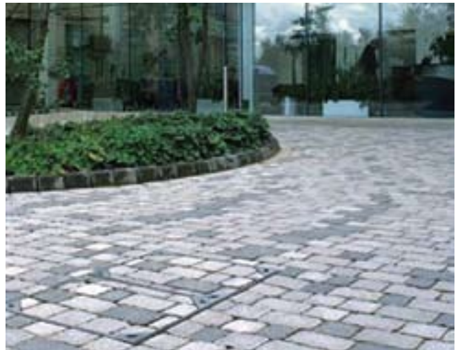
Careful selection of ironwork is essential. Here, special manhole covers have matching paving inset
