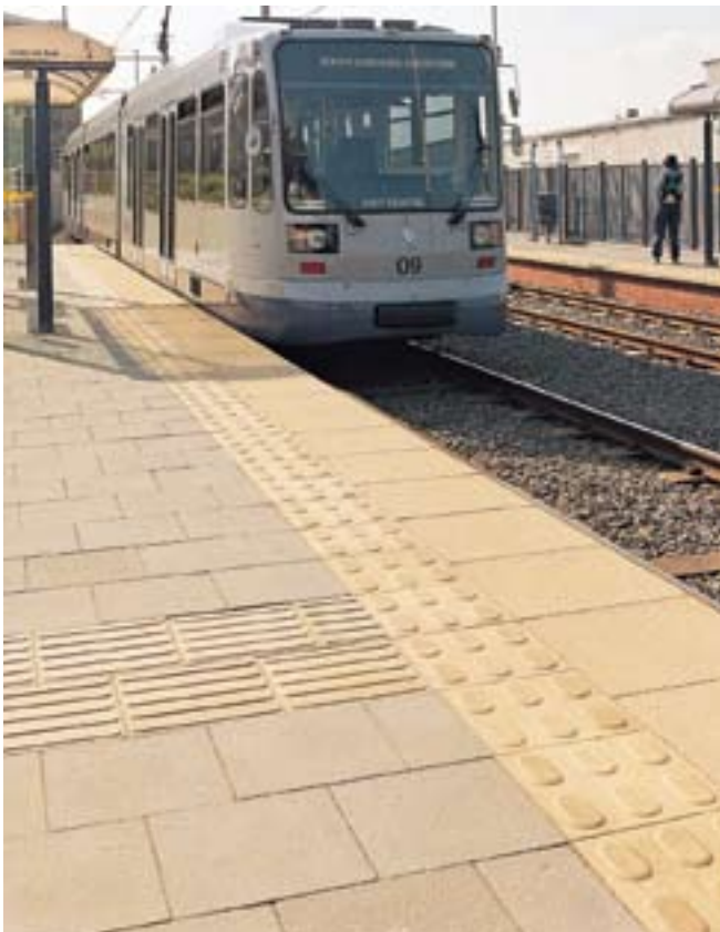
Correct use of tactile paving is essential to give the right information to visually impaired people
