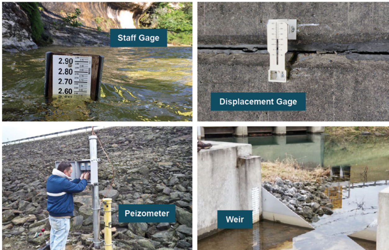
Figure 2-45: Typical Levee Instrumentation
