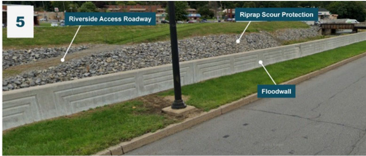
Figure 2-55: Example of Floodwall
