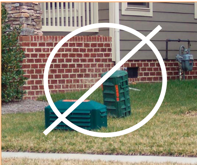
UNSCREENED OF UTILITY AND METERS ARE NOT ALLOWED
