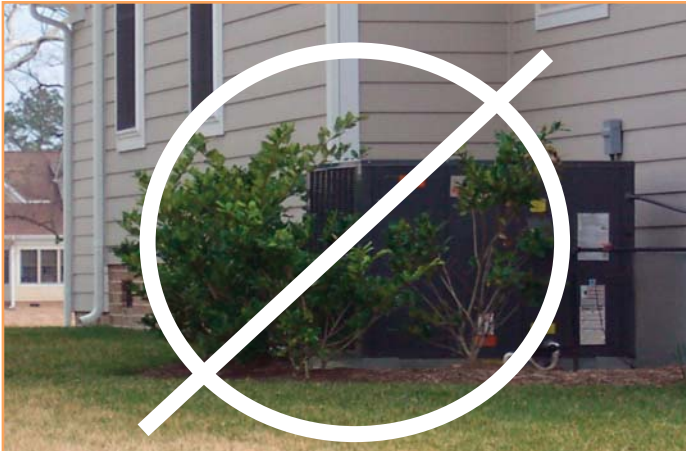
INADEQUATE LANDSCAPE SCREENING AROUND HVAC AND METERS
