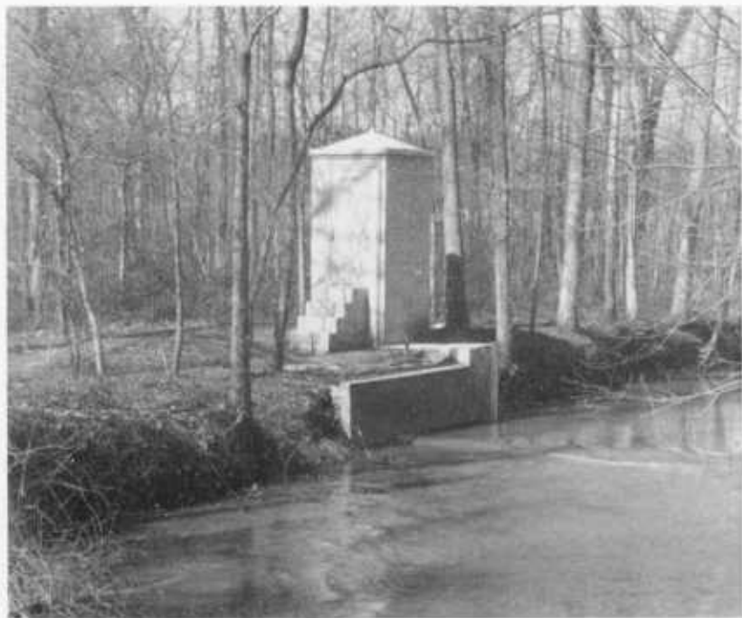
PLATE 1, FIG. 1. Gage House at Stream Flow Measurement Station on Western Branch near Largo (facing upstream).
