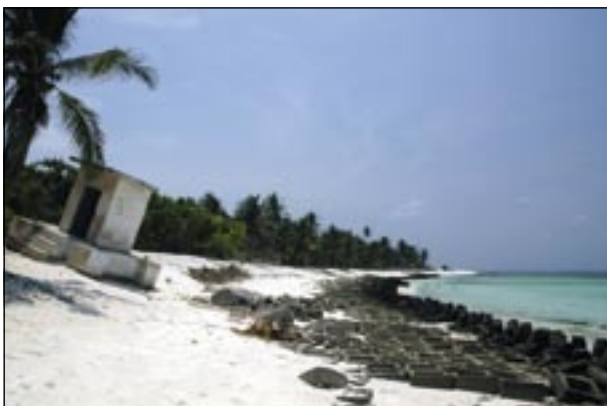
Figure 9. Cement tetrapods and other modules deployed to prevent erosion. A cyclone in 2004 caused significant loss of beach sand and infrastructure damage. Photo: JERKER TAMELANDER.
