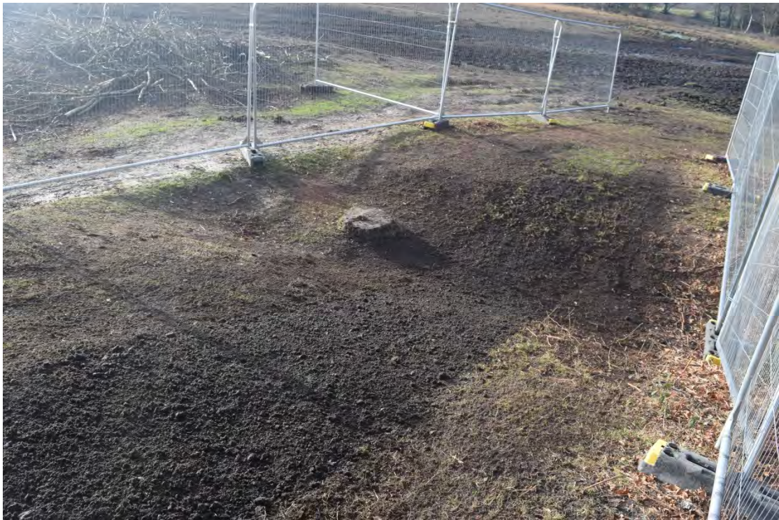
Plate 14 – General view of West end of site following backfilling and reinstatement of damaged areas. Facing SW.
