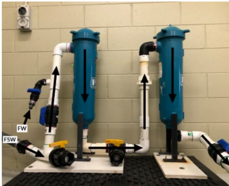
Figure 1. Pair of FSI X100 bag filter housings fitted with 1\ \mu\text{m} filter bags placed in series. Arrows indicate the direction of water flow. FSW; filtered seawater and FW; freshwater. FW is used to flush the system when cleaning.
