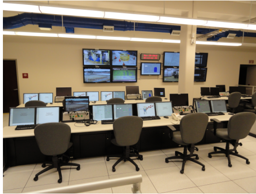
Figure 3: The modernized control room for B-2. Graphical user interfaces (GUI) for the programmable logic control (PLC) based system are visible in the foreground. Along the back wall, video monitors display test site camera images.
