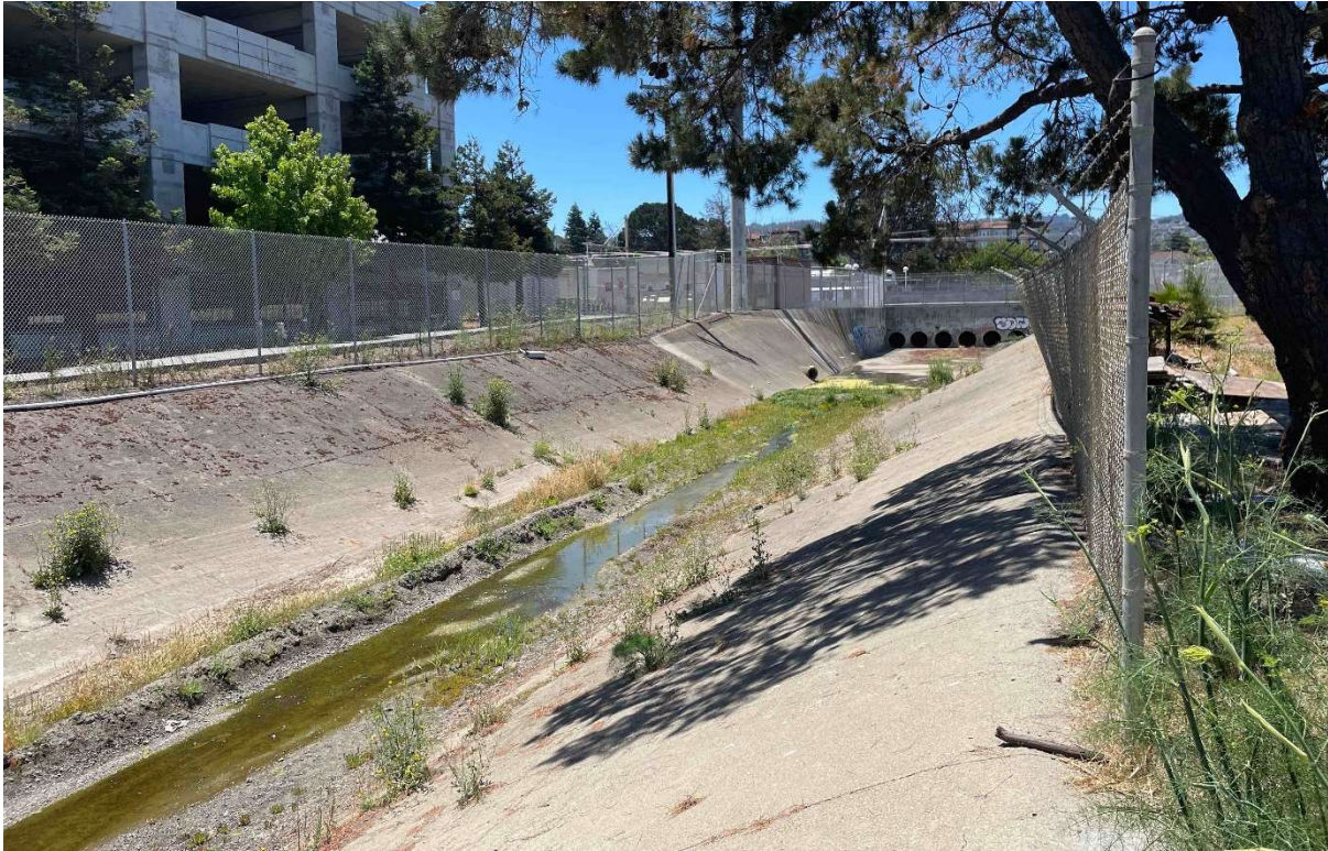
Photograph 3. Portion of Highline canal with freshwater marsh in concrete lined canal. Photo facing southwest.
