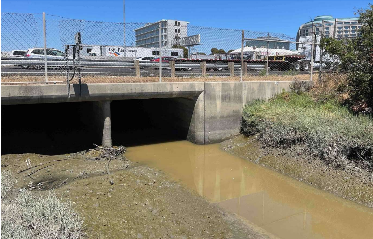
Photograph 7. View of Mills Creek as it runs under U.S. 101. Photo facing east.
