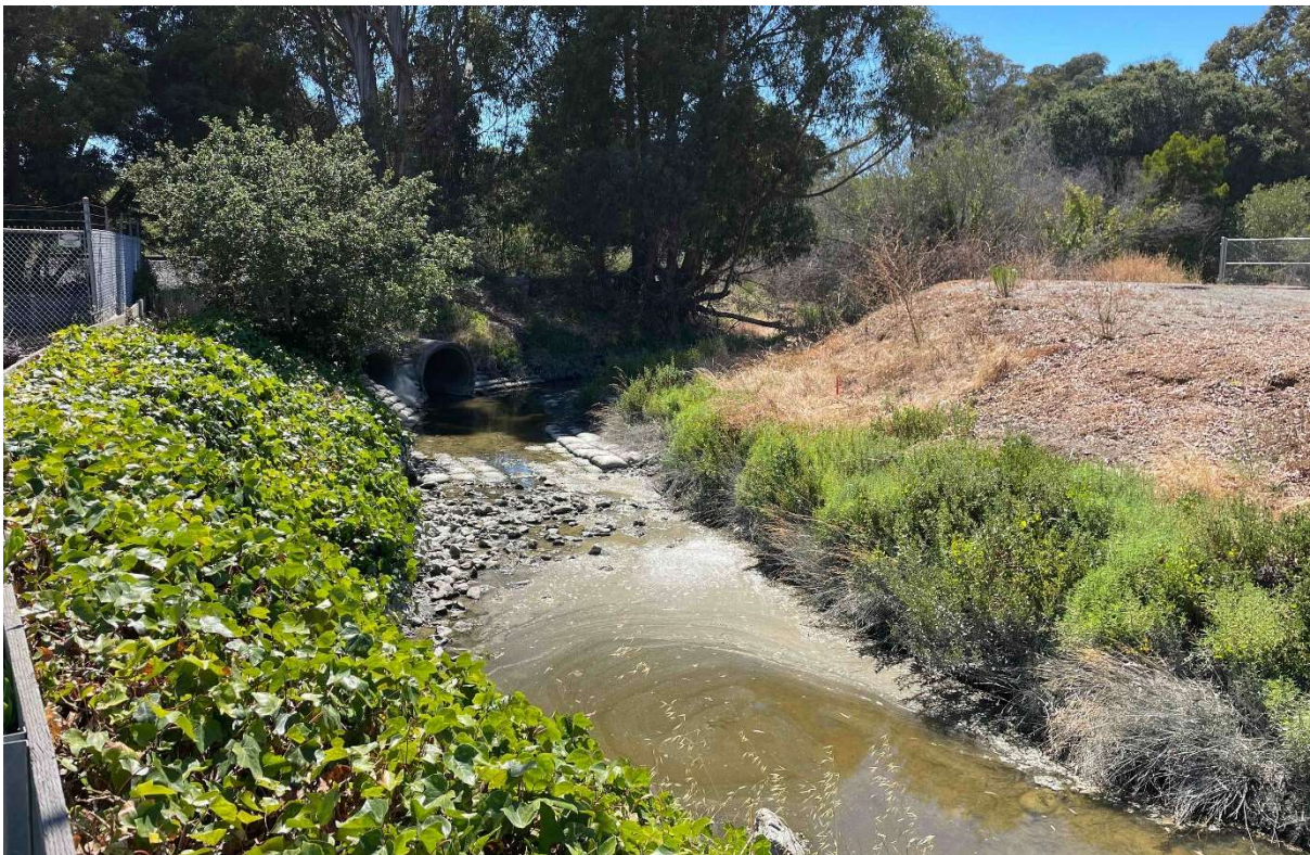
Photograph 10. View of culverted portion of Mills Creek near Rollins Road in Burlingame. Photo facing west.
