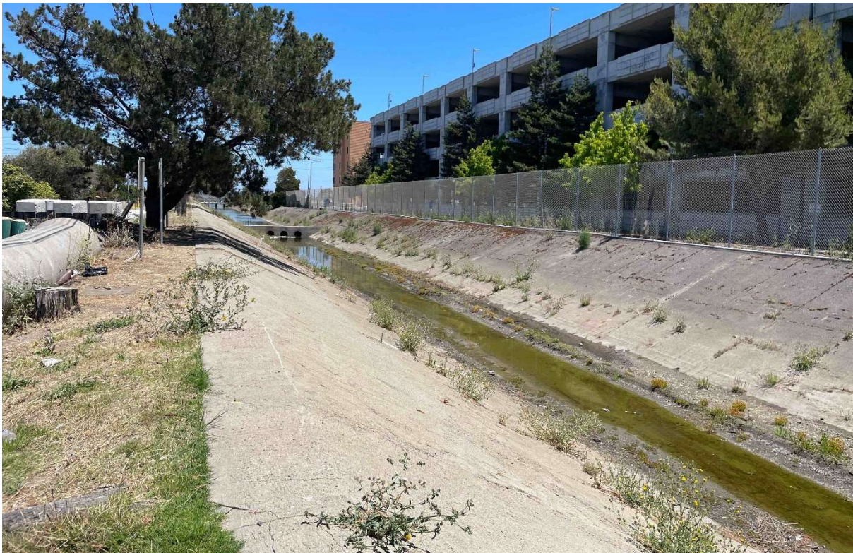
Photograph 2. View of culverts placed in concrete lined Highline Canal. Photo facing east.
