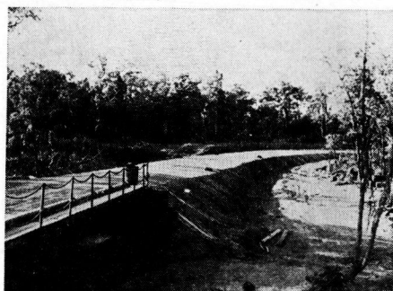
Figure 19. Tamu-Kalewa Road—Burma Protective P.B.S. Covering over Soil Grade against Erosion During Monsoon Floods
