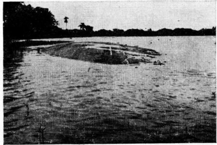
Figure 13. Flooded P.B.S. Taxiway. Note How Air, Forced Out of Subgrade by Rising Watertable Inflated the P.B.S.
