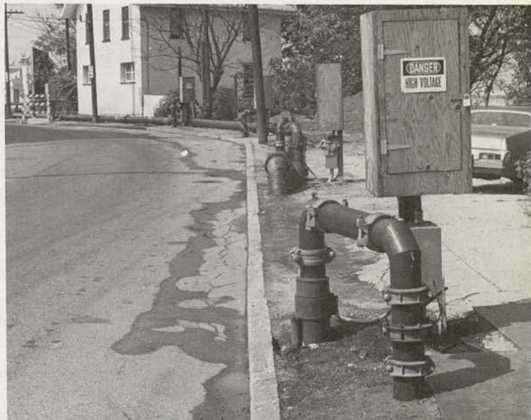
Surface pumping installation for tunnel dewatering (photo courtesy of Moretrench American Corporation).
