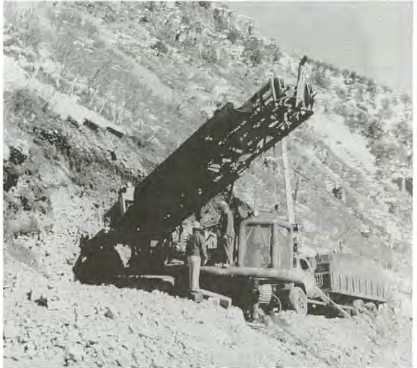
FIGURE 20-25 Large specialized rig drilling horizontal ground anchor holes in talus, Glenwood Canyon, Colorado. COLORADO DEPARTMENT OF TRANSPORTATION
