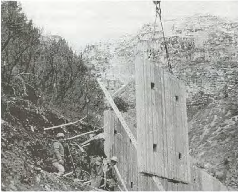
FIGURE 20-27 Installation of permanent retaining walls that utilize tiebacks into talus, Glenwood Canyon, Colorado. COLORADO DEPARTMENT OF TRANSPORTATION
