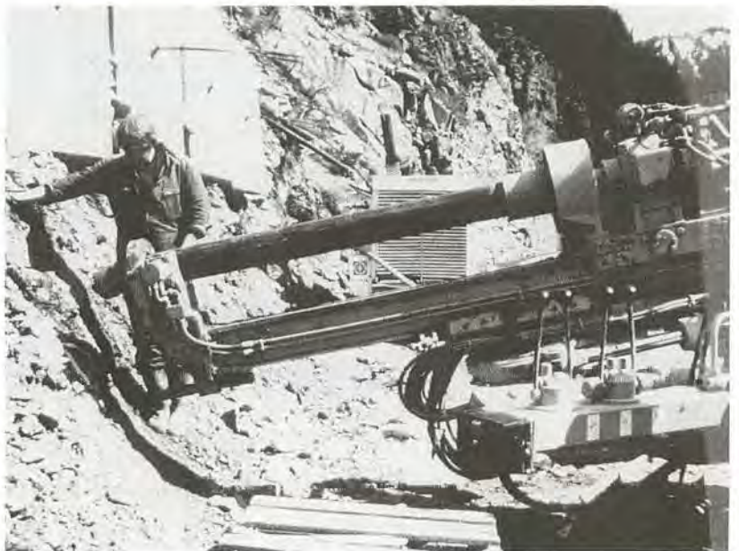
FIGURE 20-26 Smaller rig drilling ground anchor holes in talus for temporary slope-retention devices ( square concrete pads, upper part of photograph ), Glenwood Canyon, Colorado. COLORADO DEPARTMENT OF TRANSPORTATION
