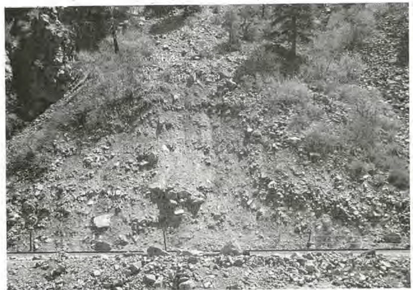
FIGURE 20-1 Colluvial slope along Denver and Rio Grande Western Railroad, Glenwood Canyon, Colorado. J.D. HIGGINS, COLORADO SCHOOL OF MINES, GOLDEN, COLORADO
