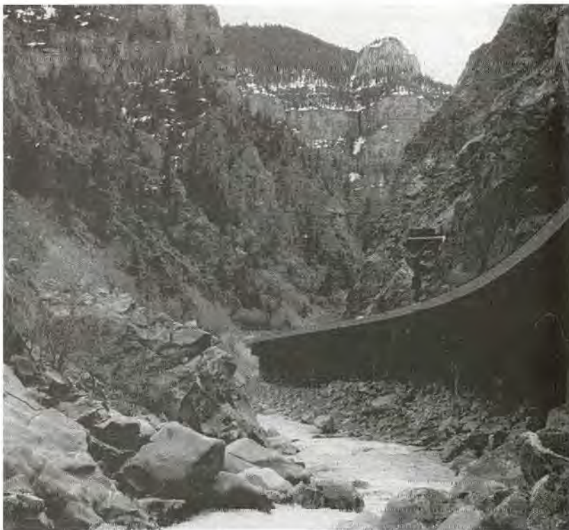
FIGURE 20-28 Interstate-70 viaduct founded on talus, Glenwood Canyon, Colorado. J.D. HIGGINS, COLORADO SCHOOL OF MINES, GOLDEN, COLORADO
