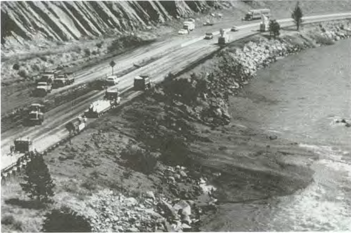
FIGURE 20-18 Cleanup activities after debris flows blocked Interstate-70 west of Glenwood Springs, Colorado. These debris flows occurred with first heavy rains after large forest fire had affected slopes above roadway. BOB ELDERKIN, BUREAU OF LAND MANAGEMENT
