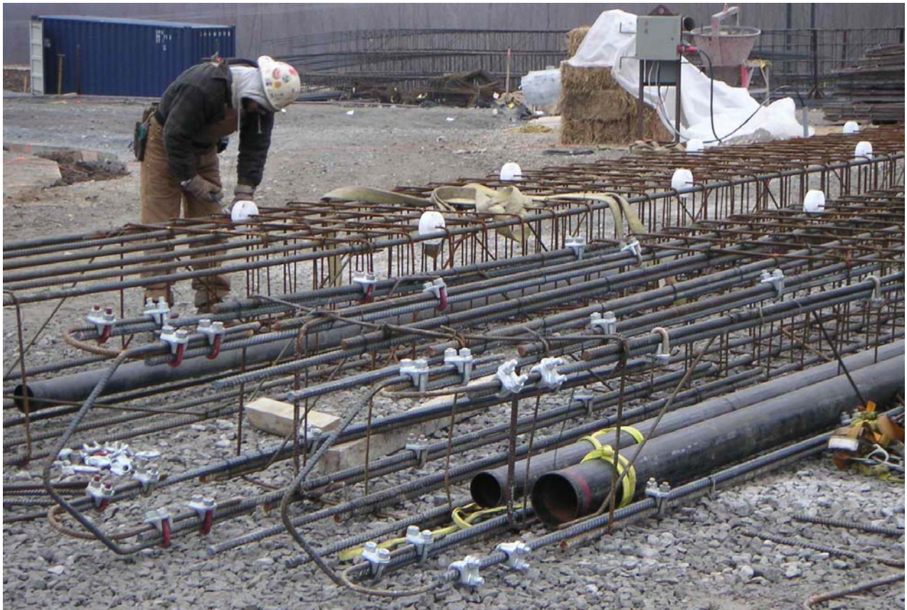
FIGURE 14 Eight-inch steel pipe placed within diaphragm wall reinforcement for housing inclinometer casing (Case Foundation Co.).
