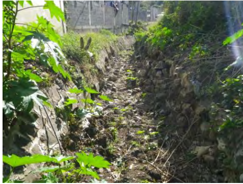
Photo 5.2.3 Seen below the Blockage No much difference from previous can be seen.
