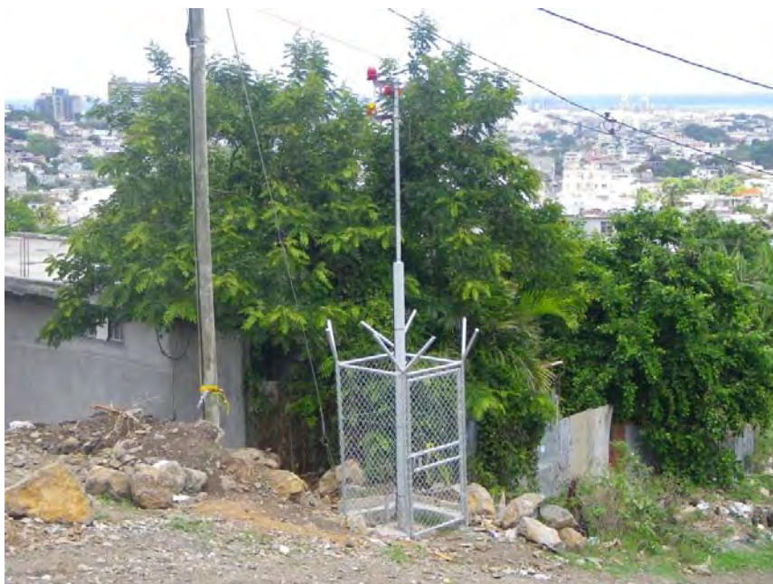
Figure 6.2.16 Installation of the Early Warning and Evacuation System in Vallee Pitot (source: JET)
