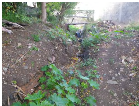
Photo 5.2.1 Upper Side of the Blockage of the Canal
