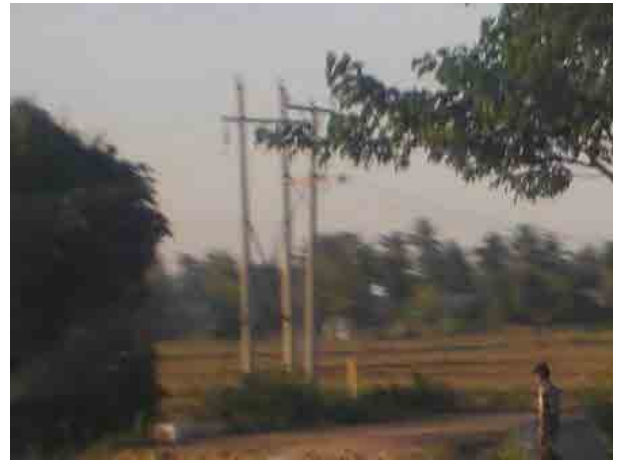
Branch off point of 33kV line
