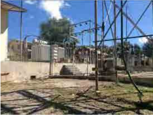
Taunggyi No.2 Substation (33/11kV, 12MVA)
