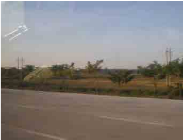
33kV transmission line
