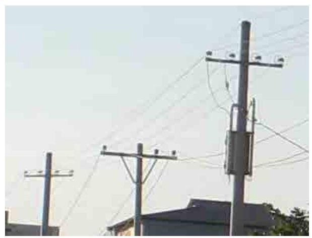
400V line and Watt hour meters on pole
