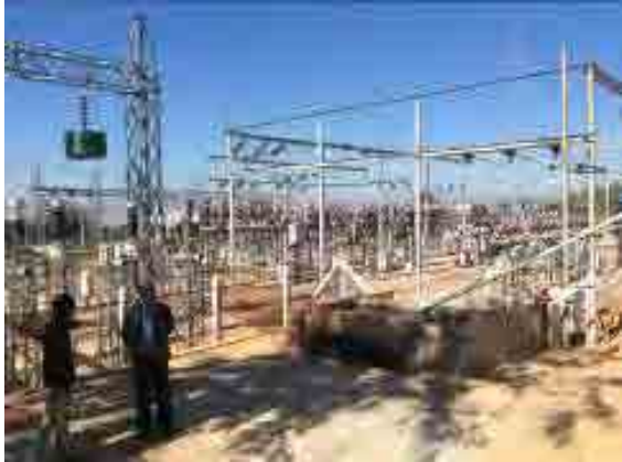
66kV/33kV Aung Sa Pye Substation
