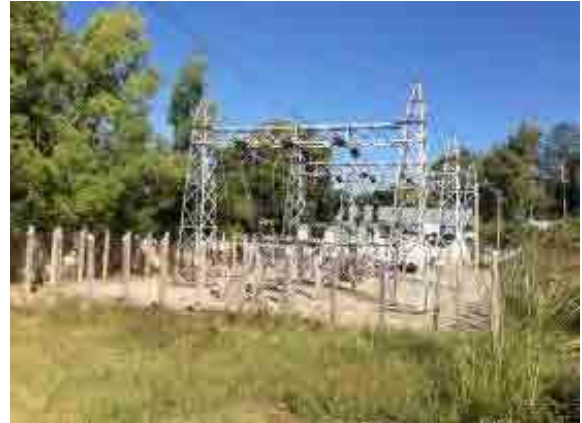
Taunggyi No.1 Substation (33/11kV, 10MVA)
