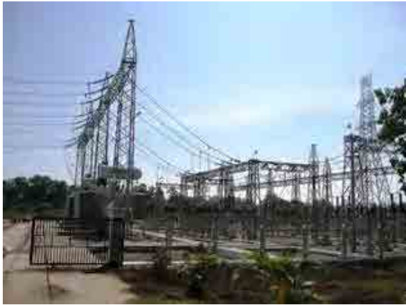
230kV Mawlamyine Primary SS
