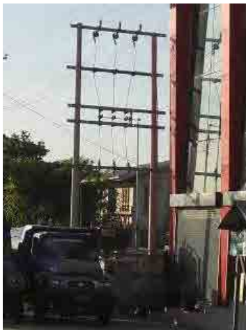
11/0.4kV Distribution transformer
