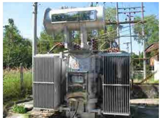
33/11kV 10MVA South SS
