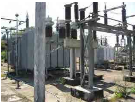
66/33kV 30MVA and 66/11kV 10MVA in Mawlamyine SS
