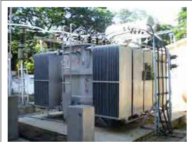
33/11kV Monywa SS (10MVA×1No.)
