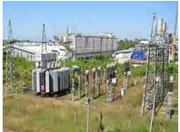
66/11kV 24MVA Nyande SS
