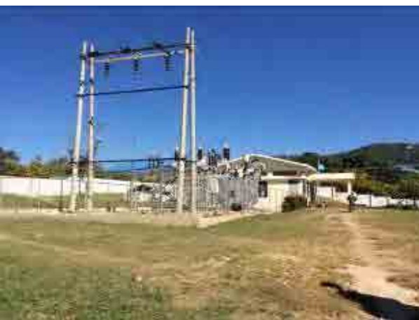
Taunggyi No.3 Substation (66/11kV, 10MVA)
