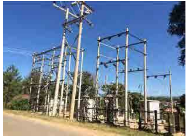
Hopone Substation (33/11kV, 5MVA)
