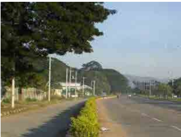
Distribution line on main street
