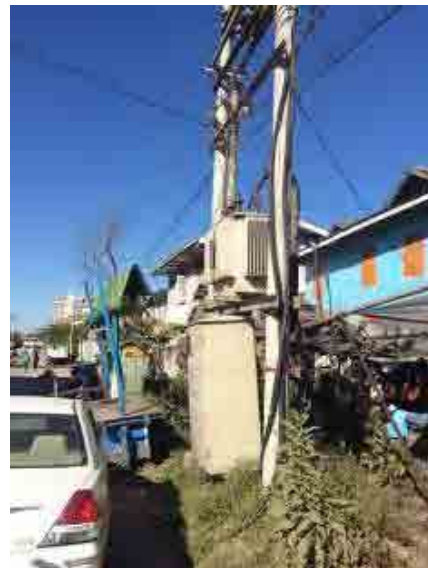
11/0.4kV Transformer in Taunggyi City
