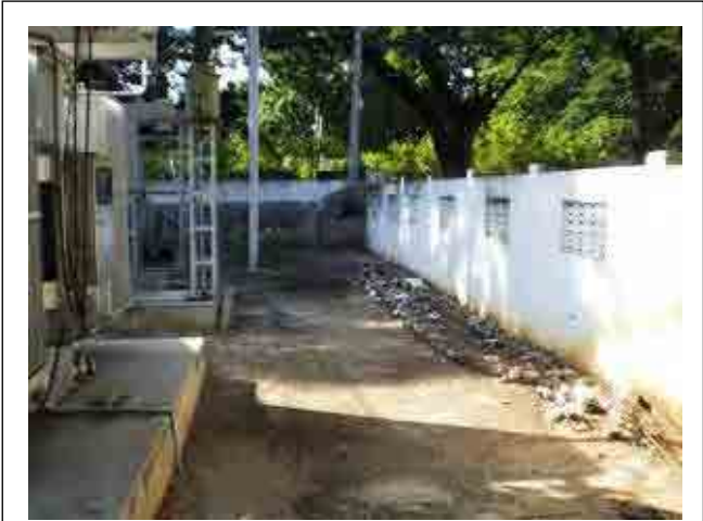
33/11kV Monywa SS Extension Area
