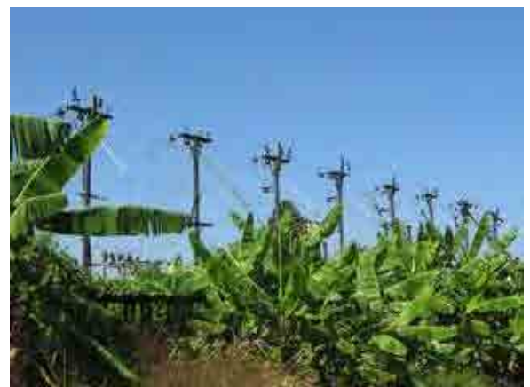
11kV feeders from Nyande SS
