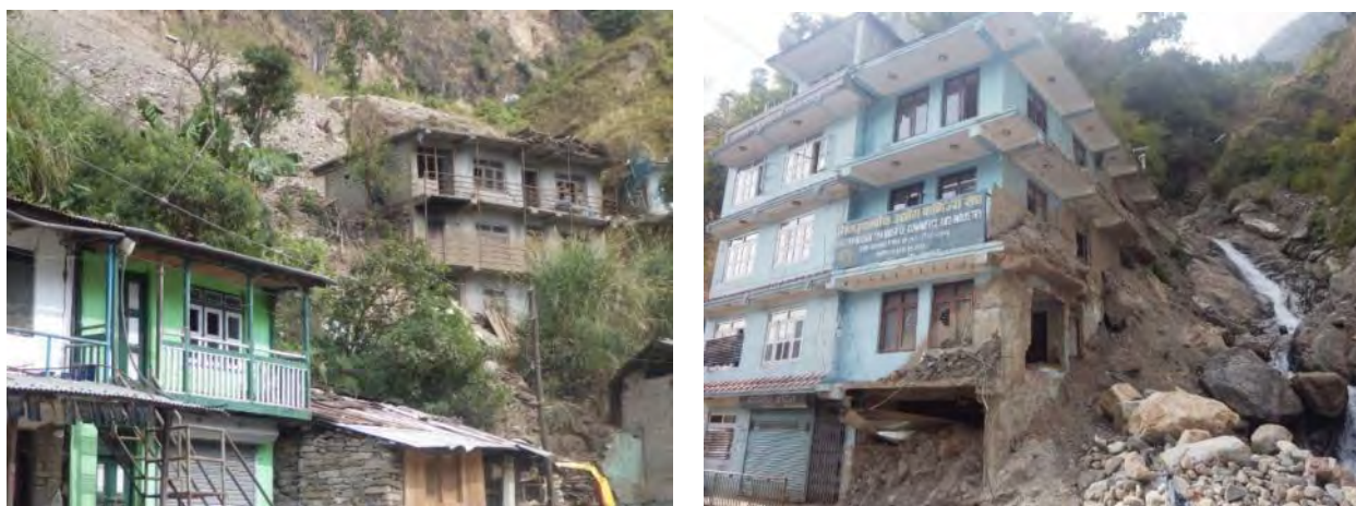
Picture 4.1 Landslide by the Earthquake in Sindhupalchowk District
