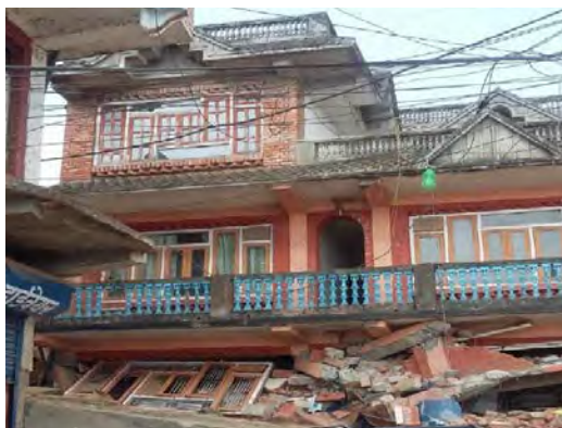
Picture 3.5 Collapsed Private House
