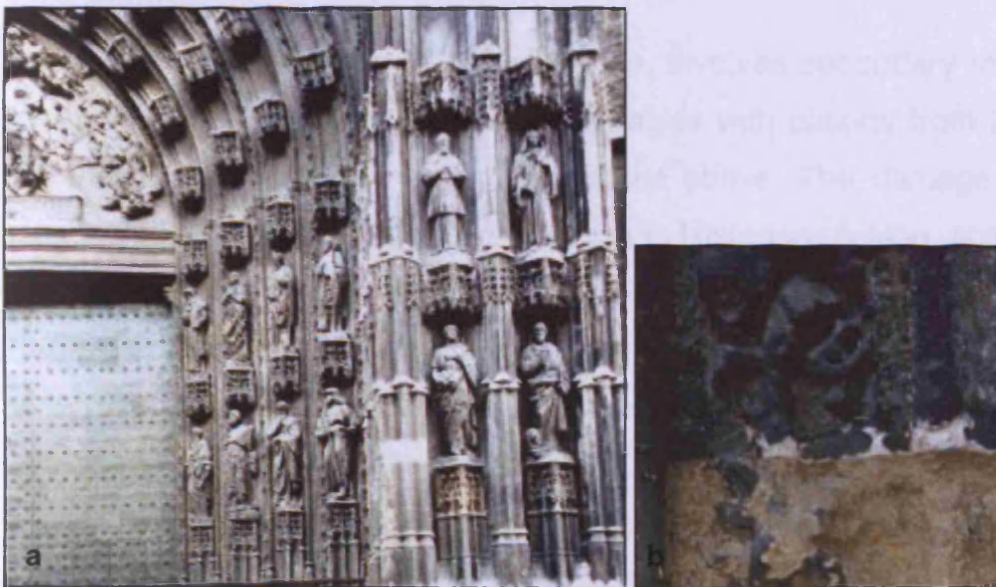
Figure 6 Black crust on Seville cathedral a. Thick black crust, with detail (b), on Seville cathedral, Spain with hydrocarbon-degrading microorganisms (Saiz-Jimenez, 1995).
