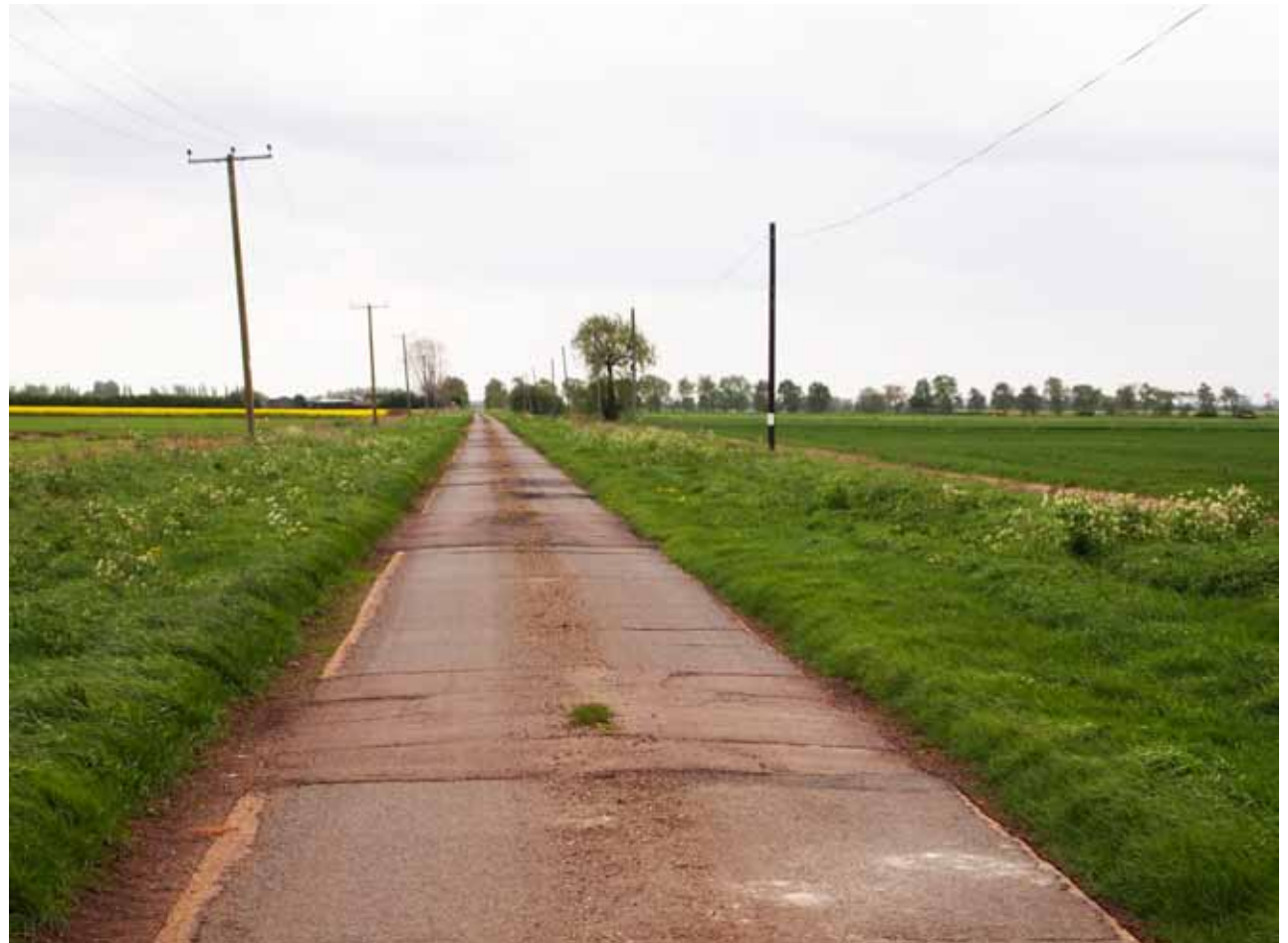
Long Drove, Haddenham - the concrete roads were laid out during the drive for intensive food productions from the land during World War II
