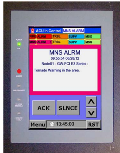
Figure 3.4.1 NGA Screen with MNS ALARM Event Displayed
