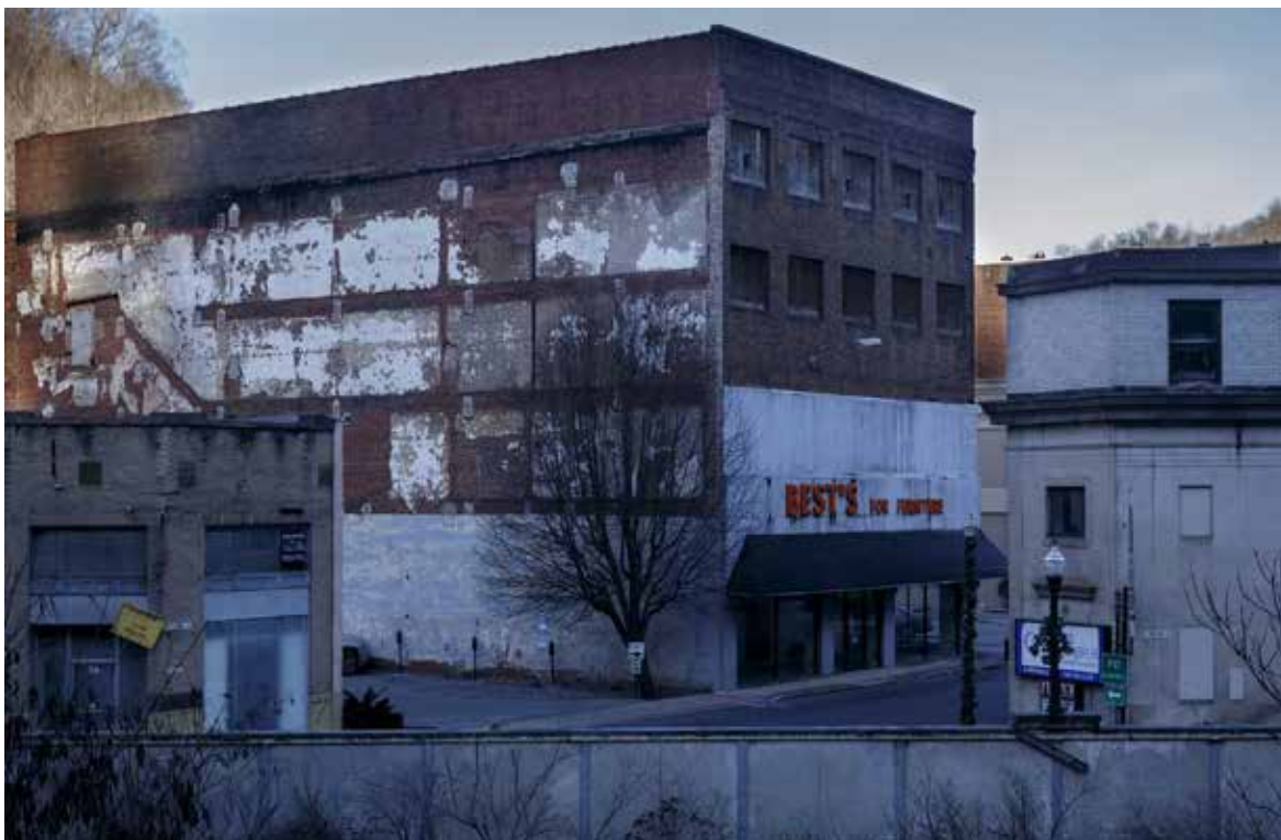
The Best's Furniture building, which will be torn down and rebuilt for the Reconnecting McDowell program, is seen in Welch. An estimated 5,000 structures in McDowell County are abandoned or condemned and need to be demolished, according to Dan Riley, the county's director of the Redevelopment Authority.
