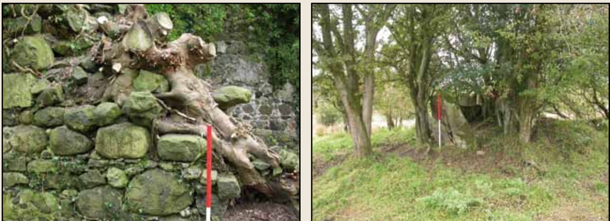
Plate 11 Magherafelt church and graveyard (LDY 042:016), showing damage caused by root action. Bullock Park portal tomb (TYR 024:029) overgrown and damaged as a consequence of root action.
