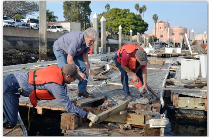
John Radovcich, Ship Carpenter for the Port of Los Angeles, directs demolition of the floating docks.
