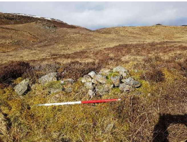
Figure 273: B170, looking NW at interior of NE gable end wall of Part B
