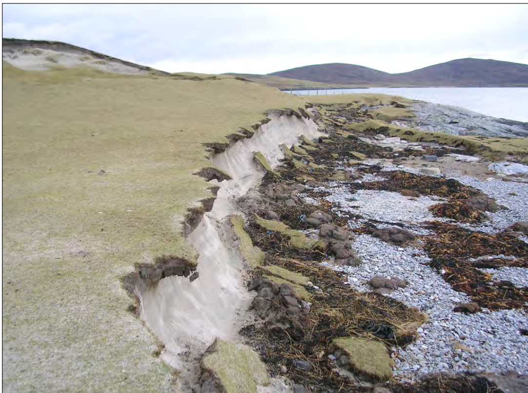
Plate 1 - Erosion causing undercutting of the coast edge, south coast of Berneray ( Coastal Geomorphology Cell 10 ).
