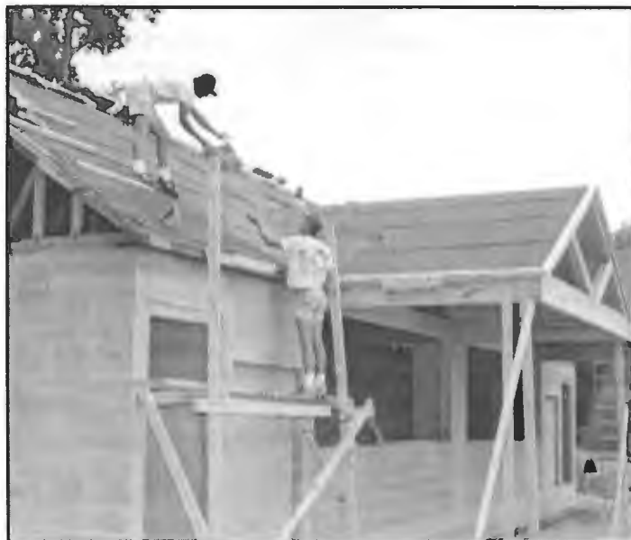
CONCESSION COMPLEX - Workers from the maintenance department at Ouachita are busy building a new concession and restroom complex at A.U. Williams Field this summer. The new facility will complement a new entrance portal to the stadium. Funding for the project was provided by the University and the Tiger Gridiron Club.
